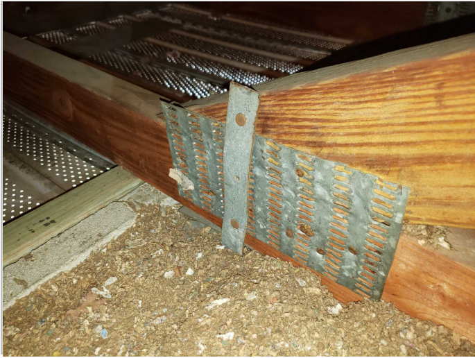
Roof to Wall: Connectors Don't Meet Requirements
