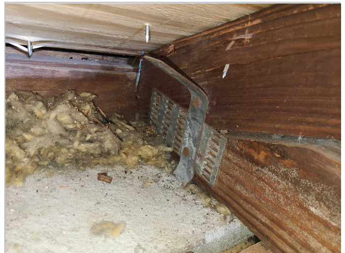
Roof to Wall: Connectors Don't Meet Requirements
