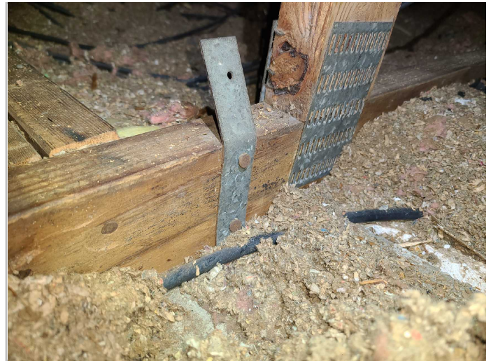
Roof to Wall: Connectors Don't Meet Requirements
