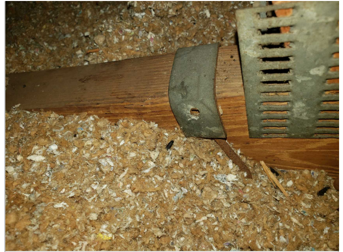
Roof to Wall: Connectors Don't Meet Requirements
