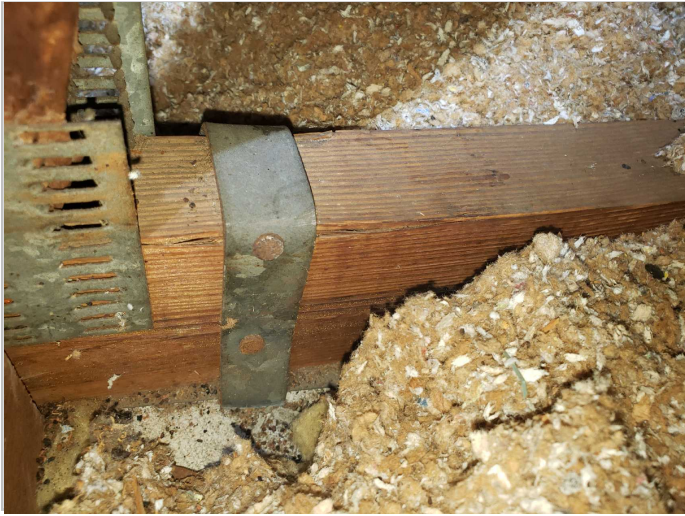
Roof to Wall: Connectors Don't Meet Requirements
