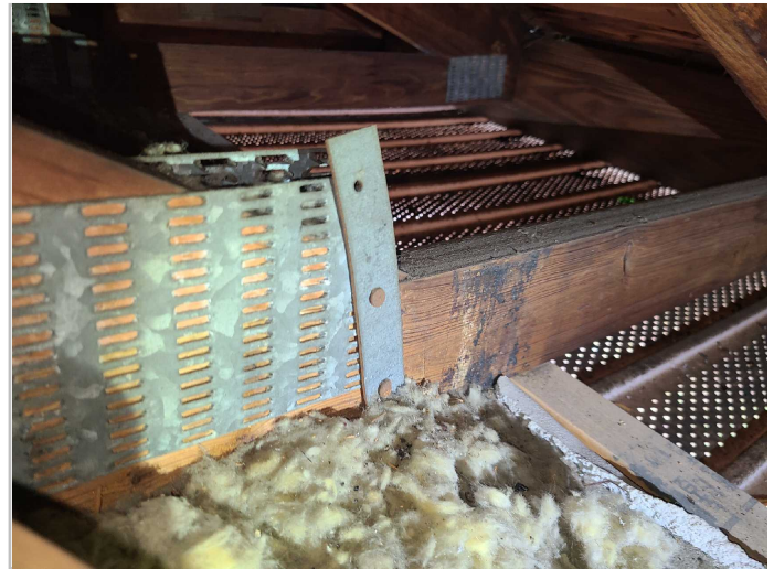
Roof to Wall: Connectors Don't Meet Requirements
