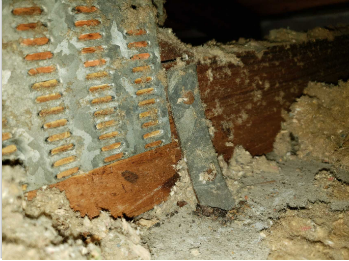
Roof to Wall: Connectors Don't Meet Requirements
