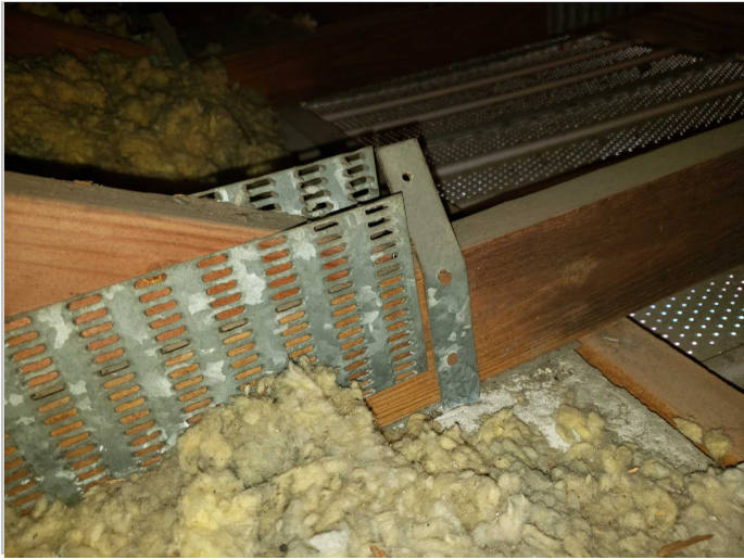
Roof to Wall: Connectors Don't Meet Requirements
