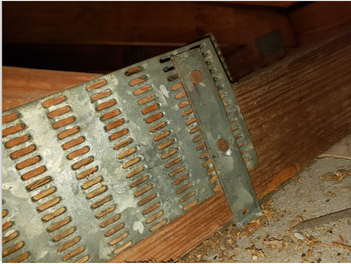
Roof to Wall: Connectors Don't Meet Requirements
