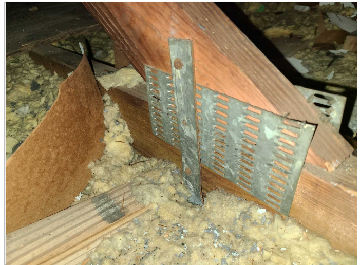
Roof to Wall: Connectors Don't Meet Requirements
