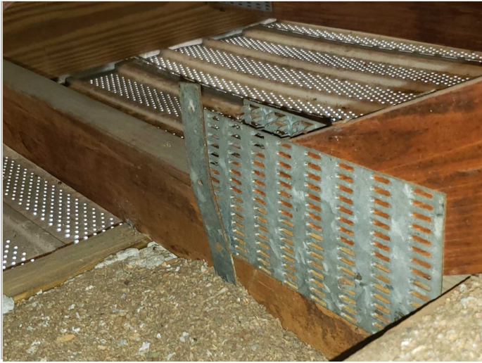
Roof to Wall: Connectors Don't Meet Requirements
