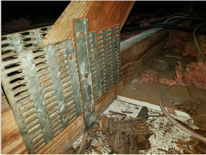
Roof to Wall: Connectors Don't Meet Requirements
