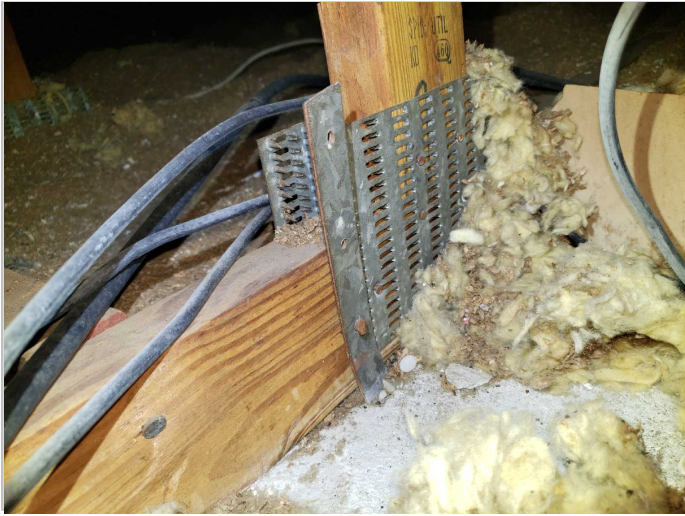
Roof to Wall: Connectors Don't Meet Requirements
