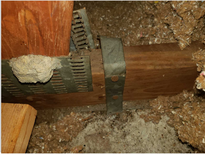
Roof to Wall: Connectors Don't Meet Requirements
