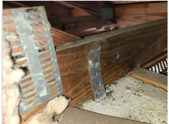
Roof to Wall: Connectors Don't Meet Requirements
